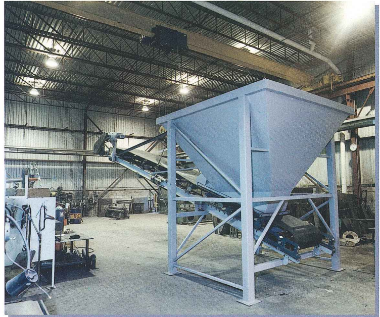
Hoppers and Material Handling Systems
